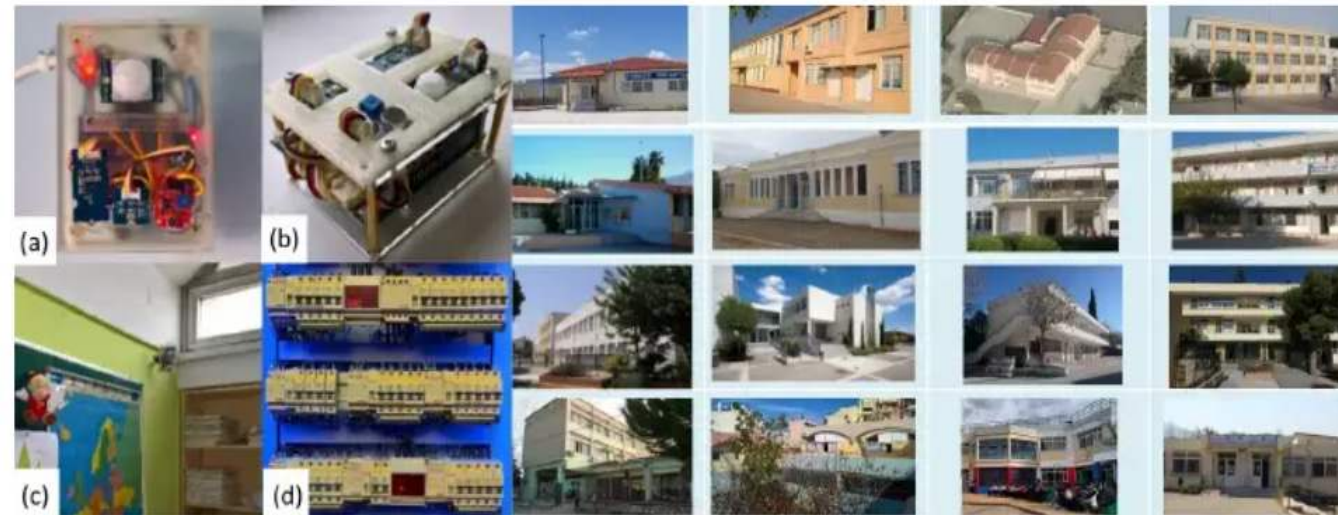
Fig. 1. Examples of the IoT infrastructure located inside school buildings in Greece (a-b) IoT nodes based on Arduino and Raspberry Pi, c) actual node inside a classroom, d) a power meter installed inside a distribution board at a Greek school, along with photos from the exterior of some of the school buildings.
